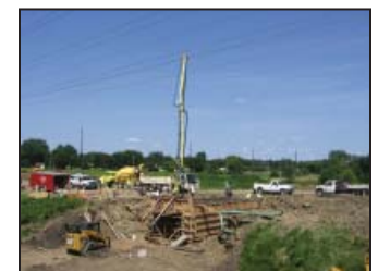
12' by 10' concrete box culvert is being constructed by Prairie Contracting south of Cherry Creek
