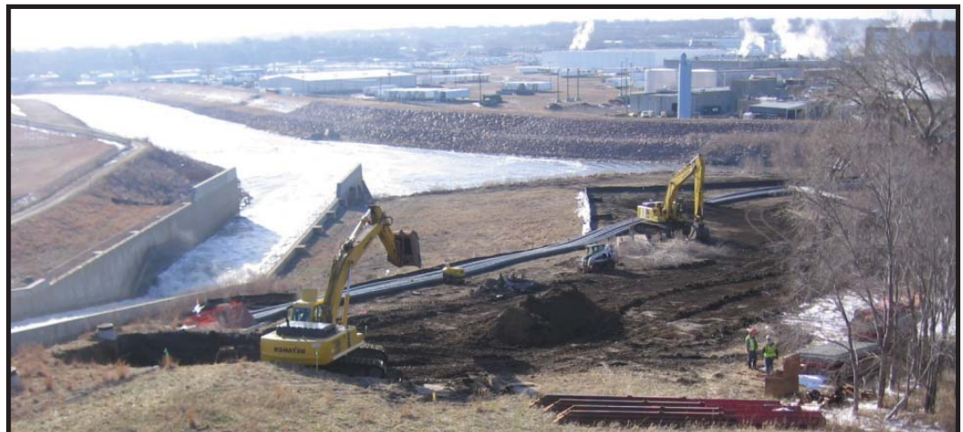
Overall view of site construction and bypass pumping piping for Segment 1 construction
