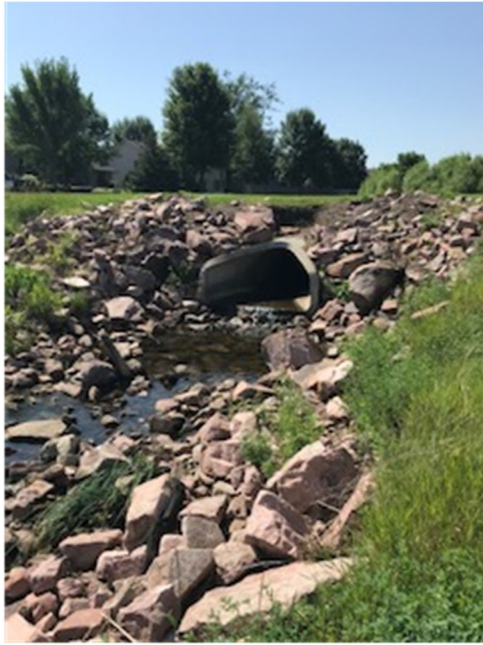
Figure 1: Erosion occurring along the southwest channel
