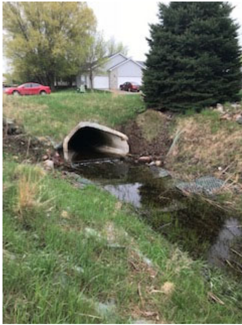
Figure 3: Erosion around culvert and channel of SE channel
