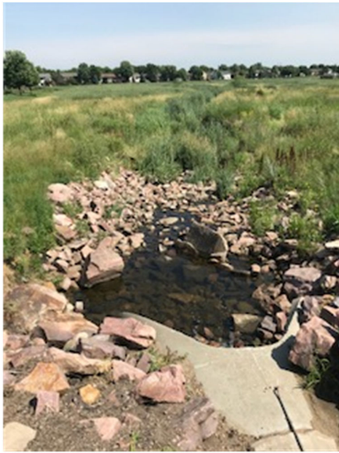
Figure 2: Erosion along the Southeast Channel
