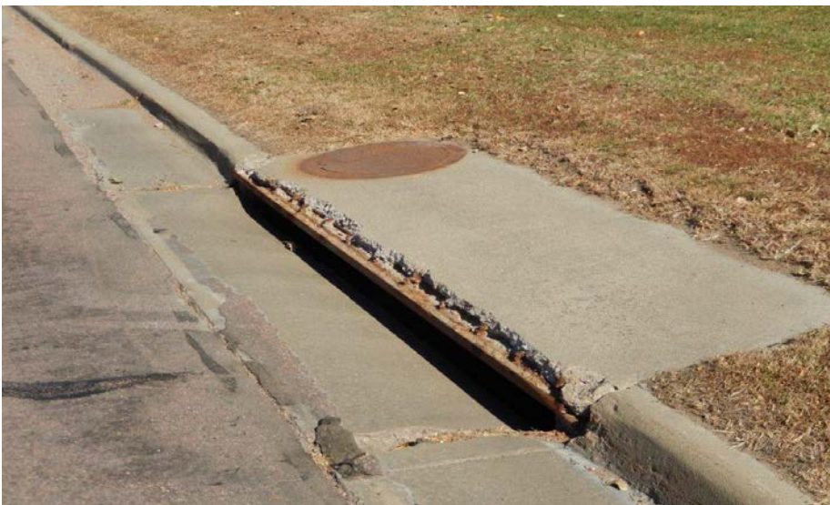
(Photo is a storm inlet in need of repairs on Southeastern Avenue.)
