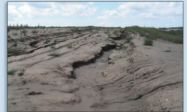
Rill and gully erosion due to no soil stabilization.
