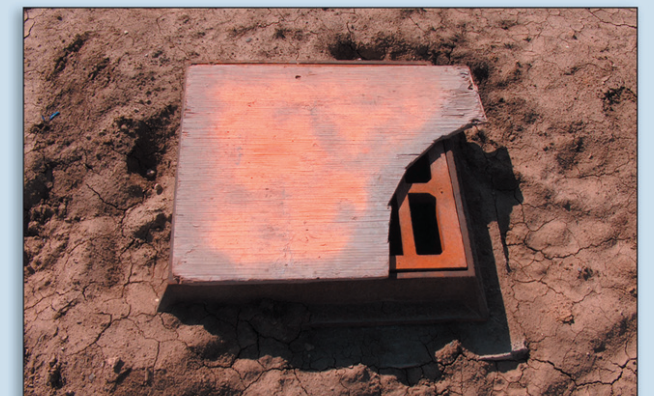
Improper stormwater inlet protection.
