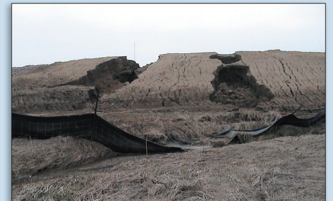
Sediment basin and silt fence failure due to no soil stabilization measures.
